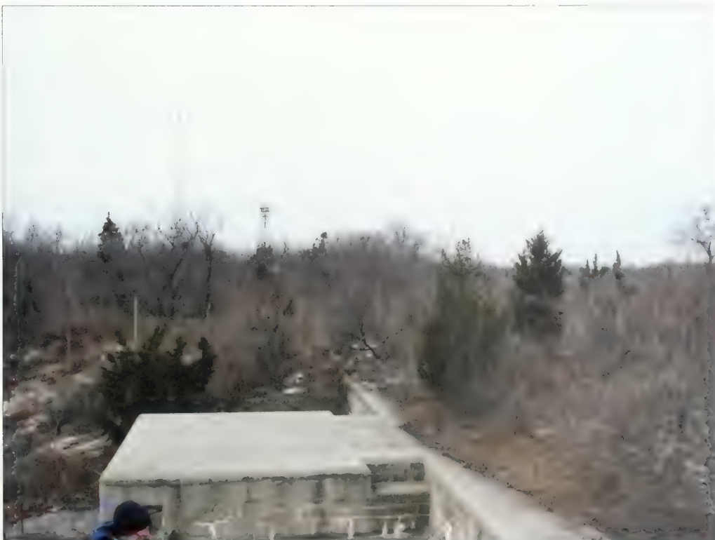
Figure 5.22. View looking west at gun platforms #5 and #6, Battery Urmston. The engineered slope meeting the concrete structure on the west and north sides contains woody vegetation growing on, or within, four feet of concrete structures and should be removed (Olmsted Center, January 2009).
